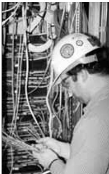
Roman TechNet cable installation foreman Dan Patterson works on one of three head end cable cabinets in the plant.
